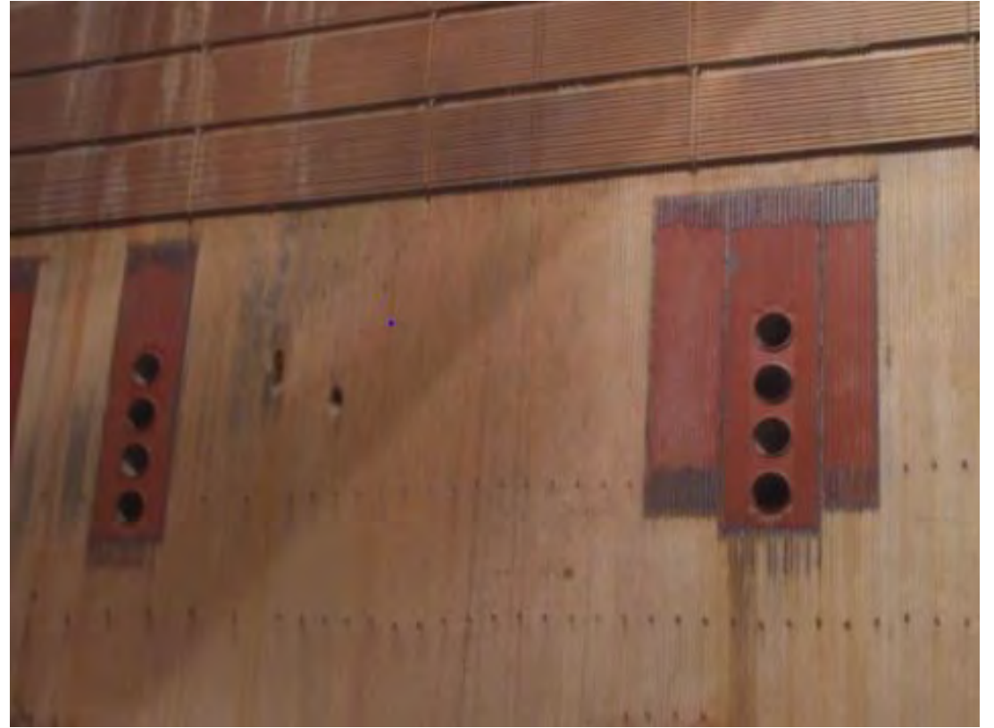
Lower Level Nozzles in Furnace
